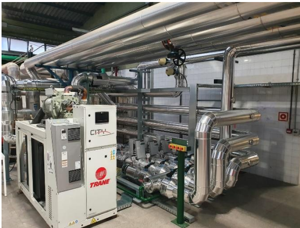
The heat pump and part of the distribution network
