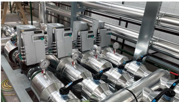
Final hot water distribution installation
