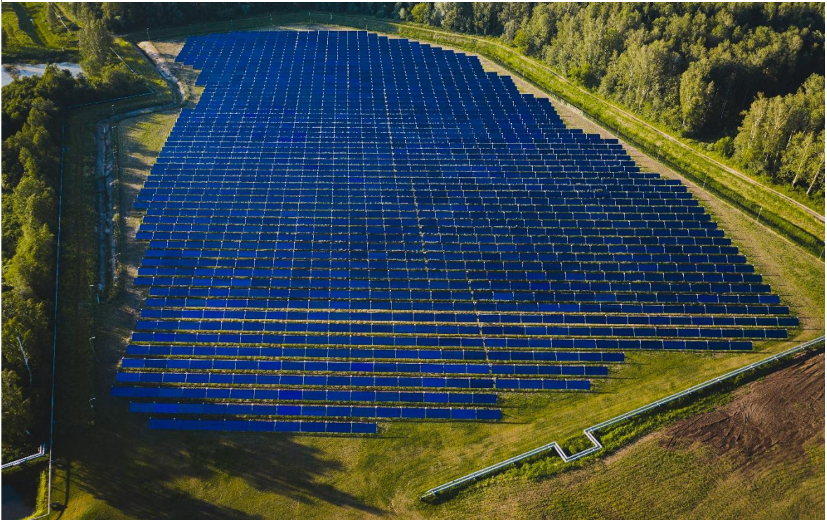
Figure 5. Bird's eye view of the solar collector field
