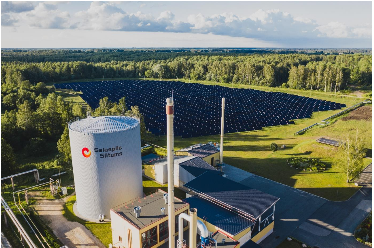
Figure 6. Bird's eye view of the solar collector field, boiler house and storage tank
