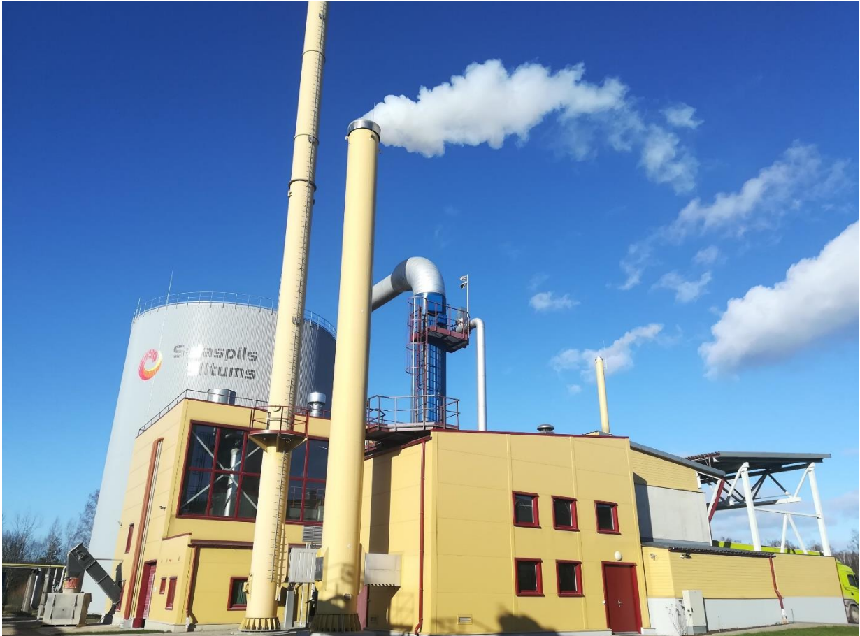
Figure 7. Boiler house and storage tank in action
