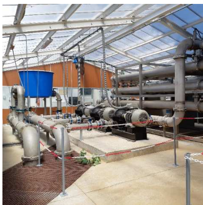
Submersible pumps at vertical shaft
