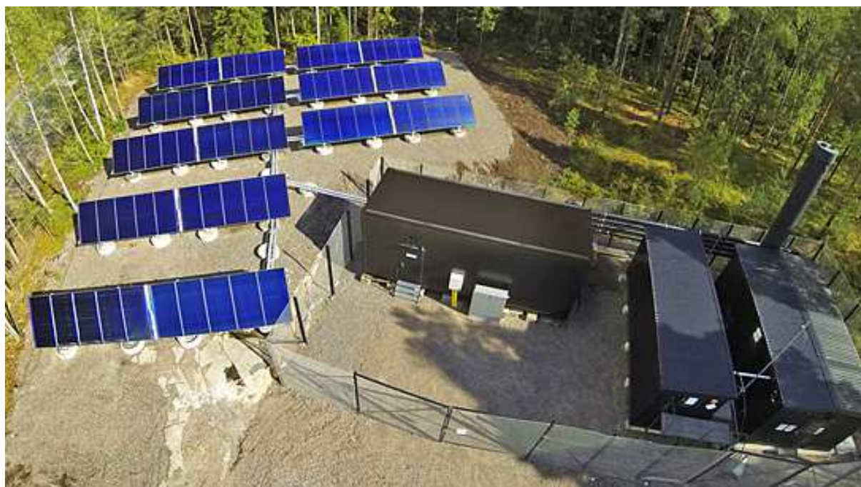
The solar collectors in the schoolyard in Sakarinmäki.
