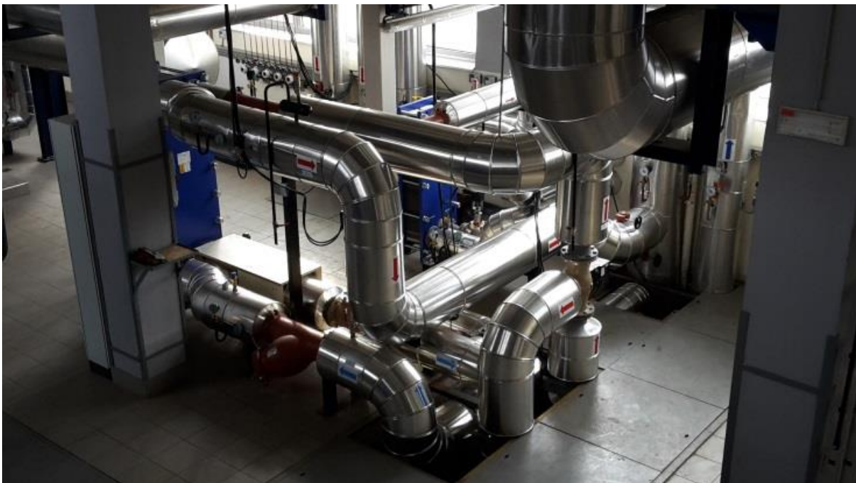
Figure 4: System for waste heat utilization in the field of district heating (Petrol Energetika)
