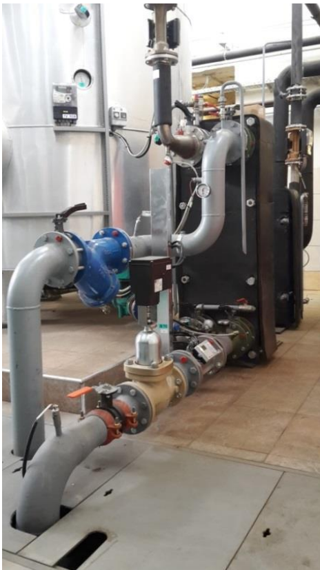
Figure 5: System for waste heat utilization in the field of sanitary hot water (Petrol Energetika)
