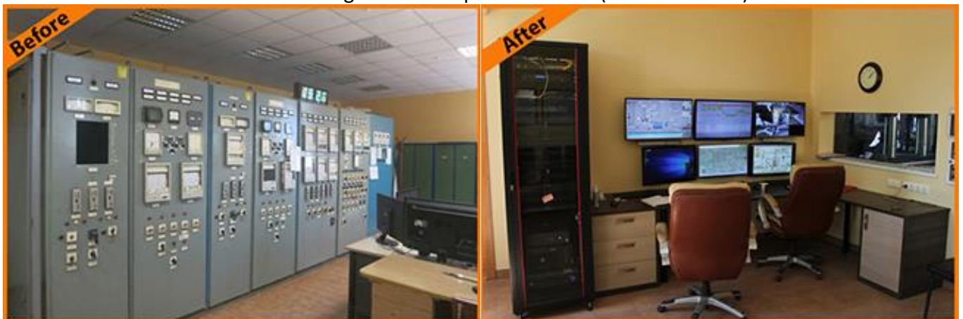
Fig 2 Heat power plant control system (2015 and 2016)
