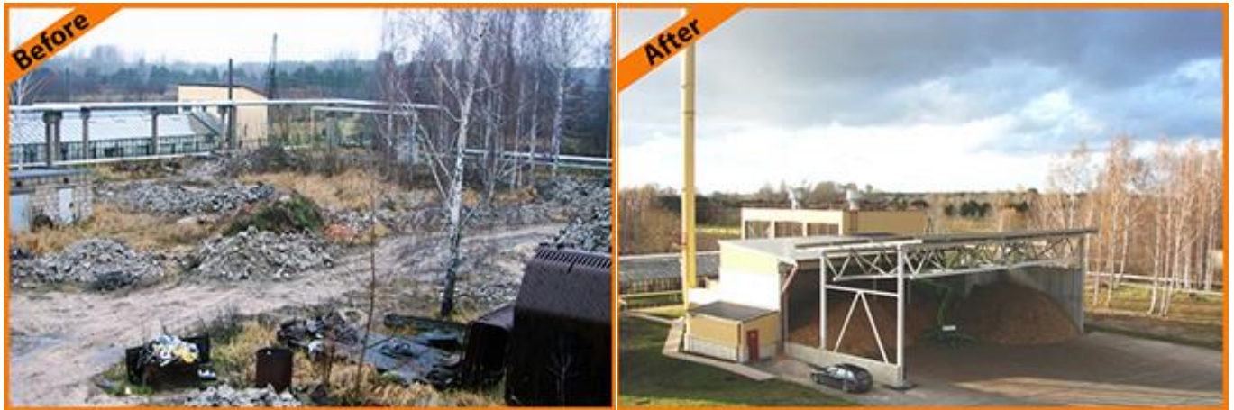
Fig. 1 Woodchip boiler house (2012 and 2016)
