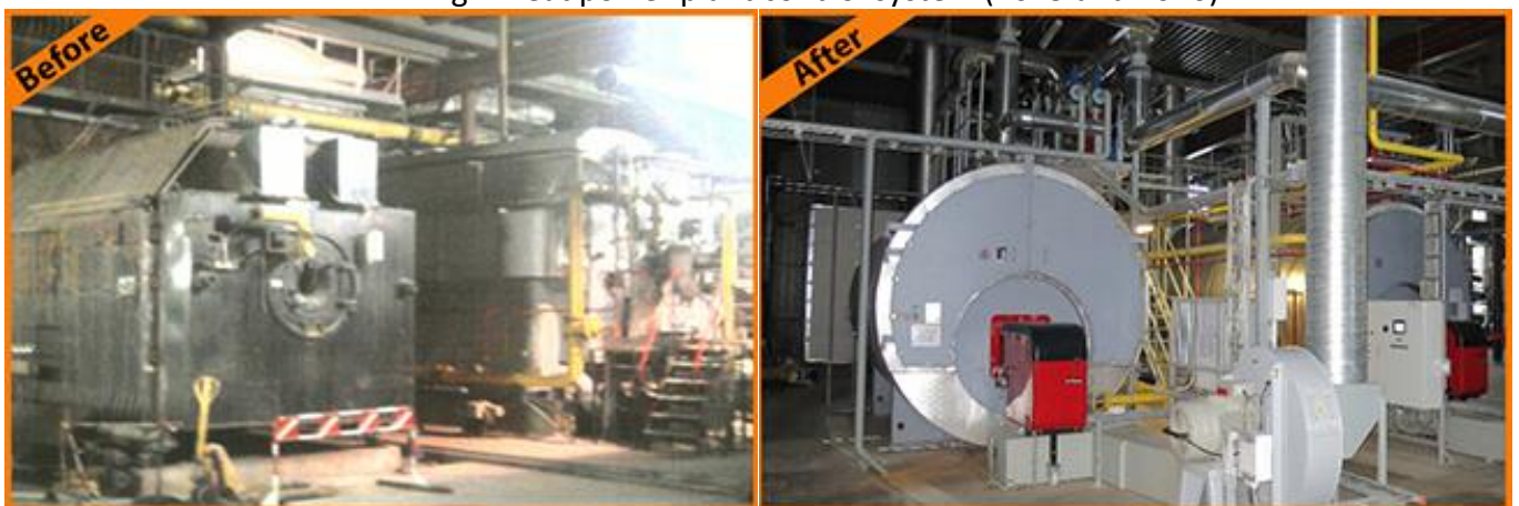
Fig 3. Gas boiler (2010 and 2016)
