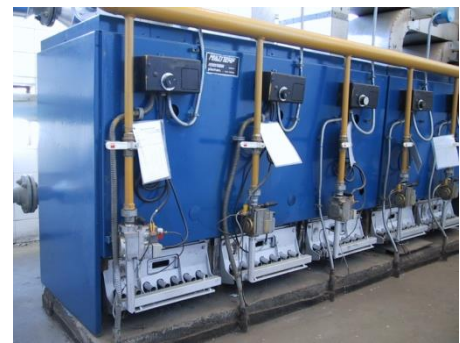
Picture No. 1: Existing boilers in a typical boiler plant
