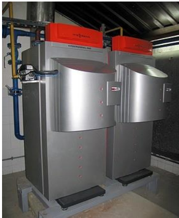
Boiler plant H4: Type Vitocrossal 300, CM3, product of Viessmann, thermal capacity 2x130 kW, made of Inox, with Matrix radiant burner and modulated regulation
