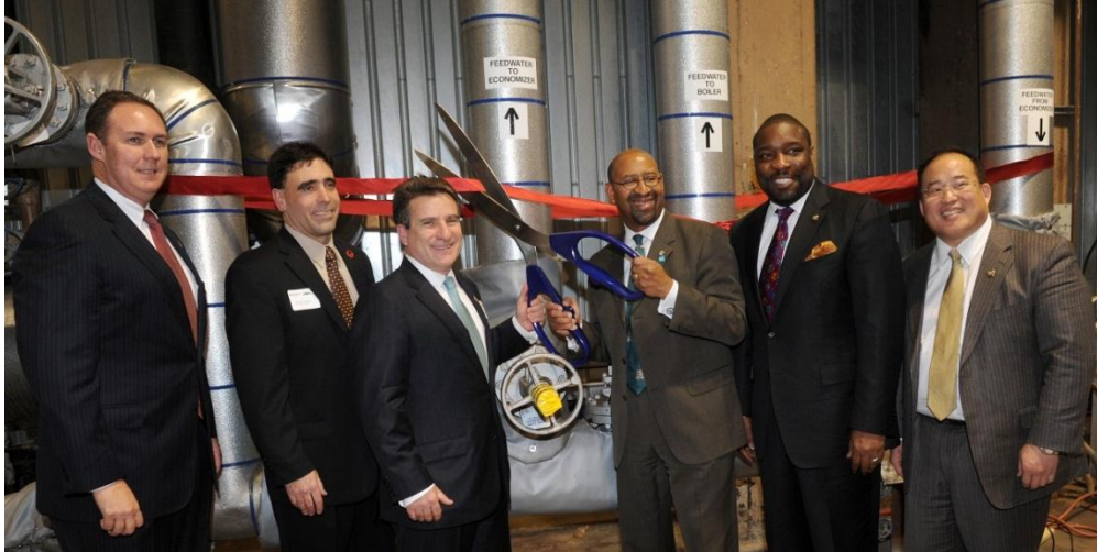
January 13, 2013: Ribbon Cutting for the Green Steam conversion
