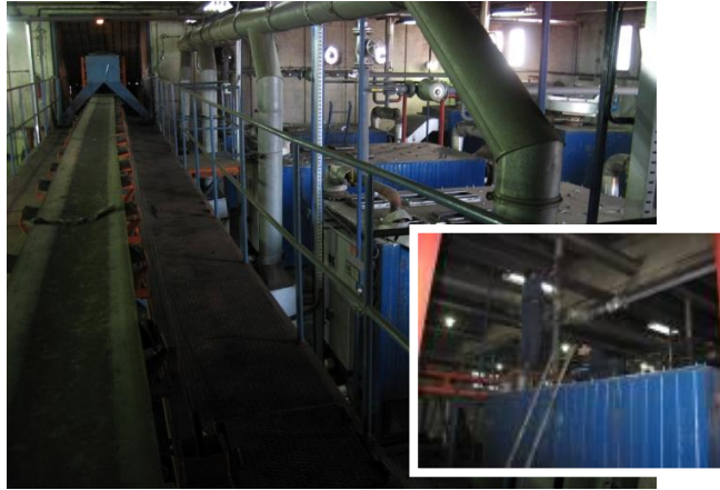
Fig. 2 Boilers and belt-conveyor.
