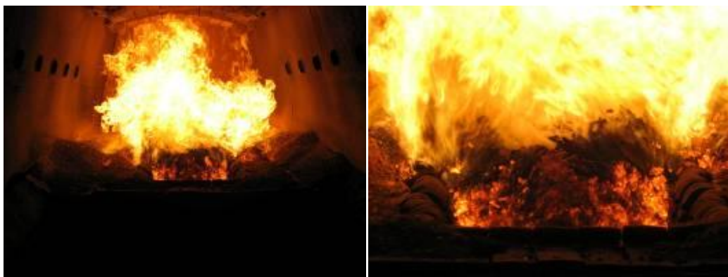
Fig. 6 Combustion of pellets, view from the open boiler door.
