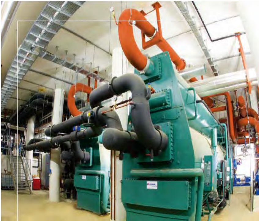
Pictures: District Cooling
