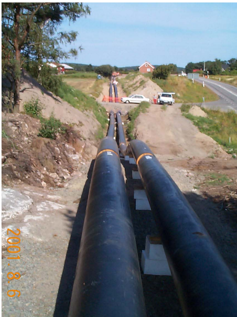
Picture 2. The heat transmission pipeline between Värö and Varberg, when constructed in 2001. Picture taken Aug 6, 2001.
