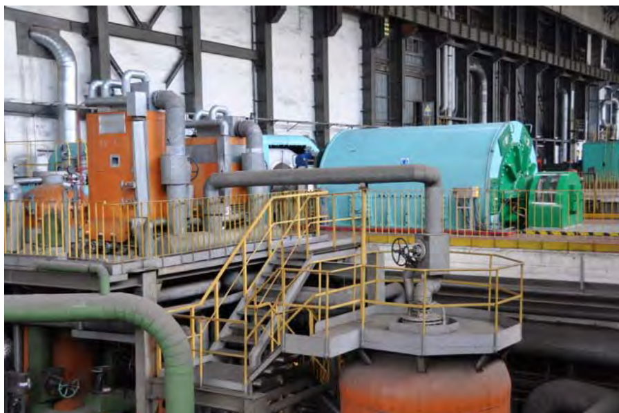
The interior of the Karolin CHP Plant engine room
