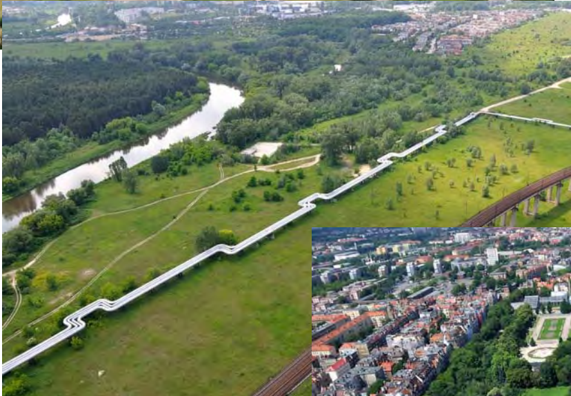
A piece of the overhead heating system providing citizens of Poznań with heat.
