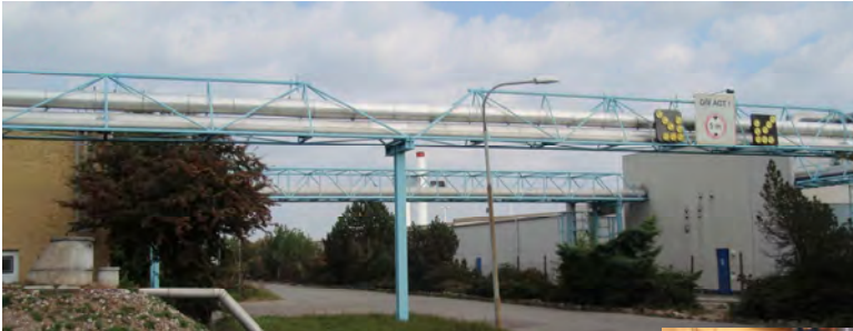
The pipes between the main heating plant and a supplier of surplus heat.
