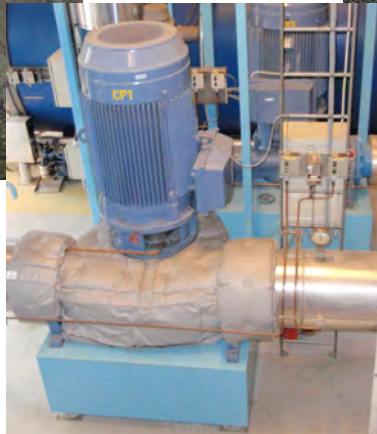
Circulating pump forwarding the district heating on to the distribution network.
