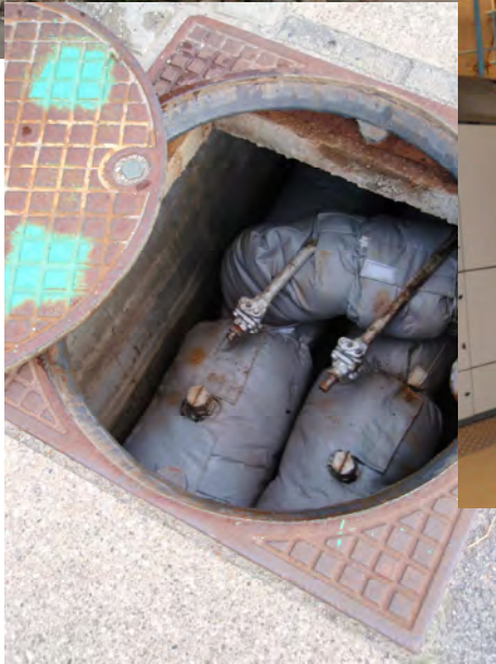
Insulated pipes in a valve well.
