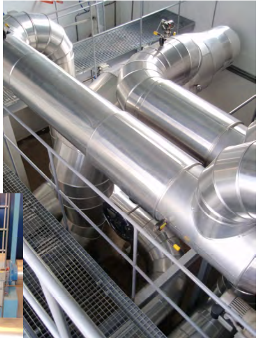
The primary well for distribution of district heating to the network.
