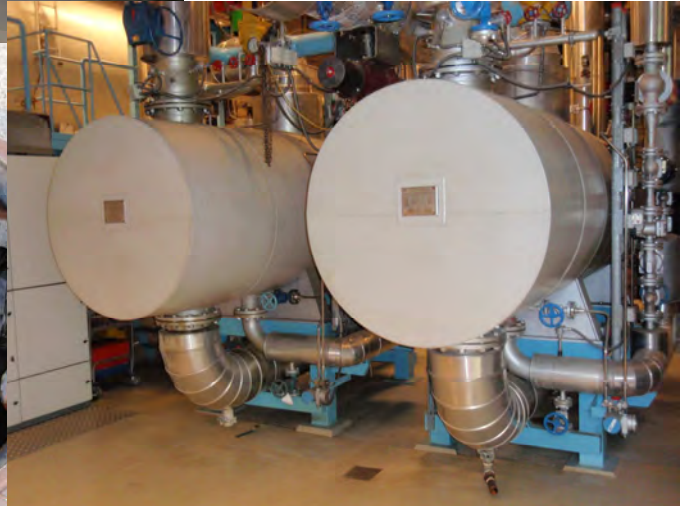
Heat exchanges on the main heating plant receives surplus heat steam from a chemical plant next door
