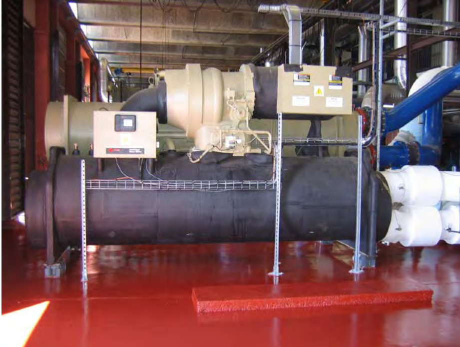
Trane centrifugal chiller with a capacity of 3600 kW
