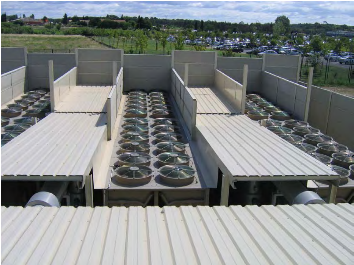
Air-cooled condenser unit
