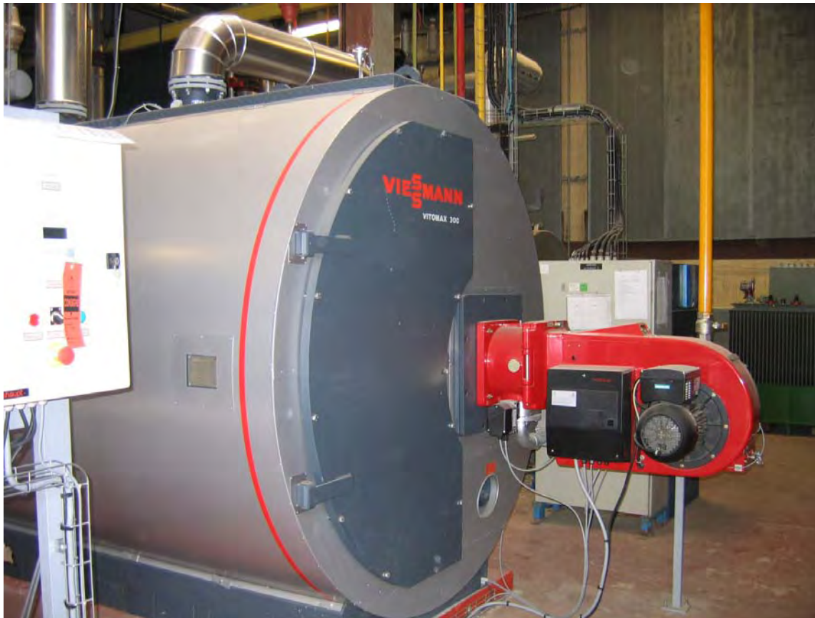
Viessmann boiler equipped with a condensate collector
