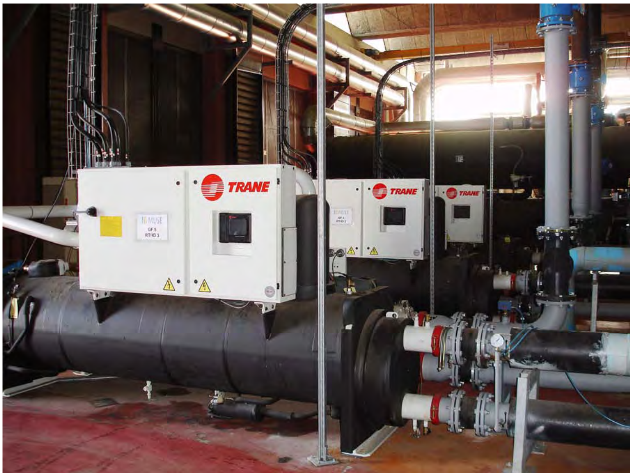
Trane heating pump (heating capacity: 1120 kW / cooling capacity: 920 kW)
