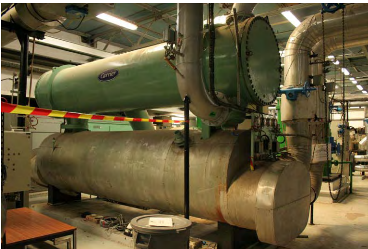
Recovered equipment Carrier brand centrifugal chiller 3500 kW
