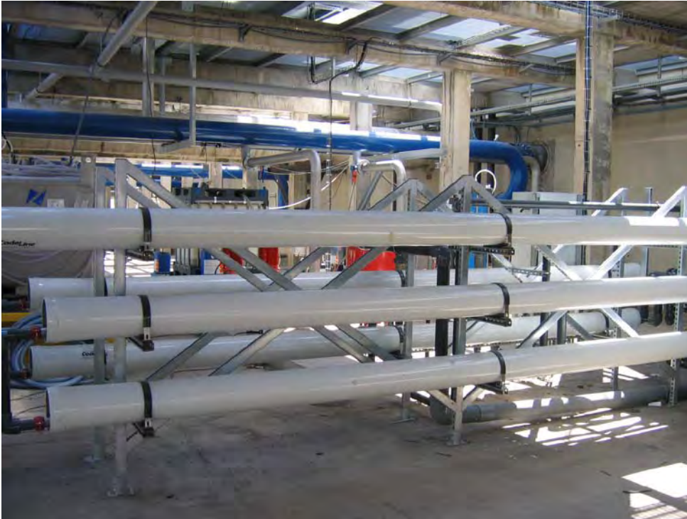
Reverse osmosis water treatment
