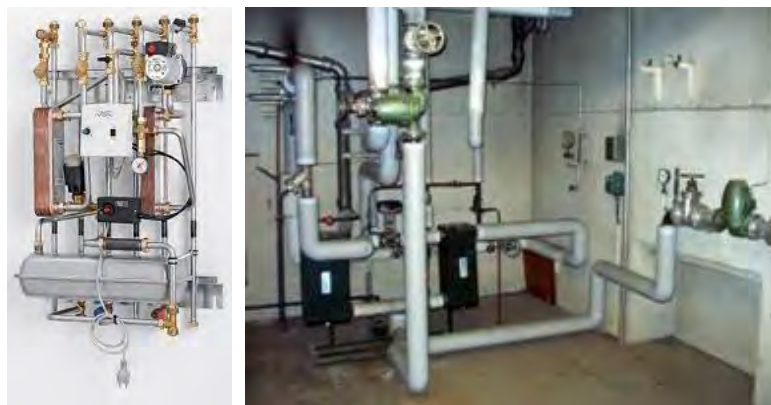
Picture 6. Typical small-scale and large-scale DH customers' installation. (Photo: E.ON)
