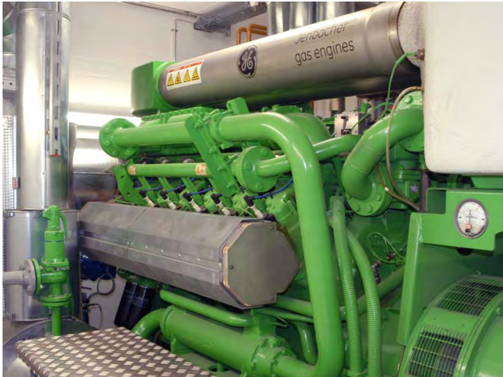
Biogas- CHP-unit, 624 kWel
