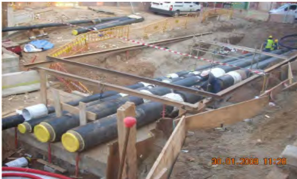
Fig.8: View of a ditch with cold and hot water pipes.
